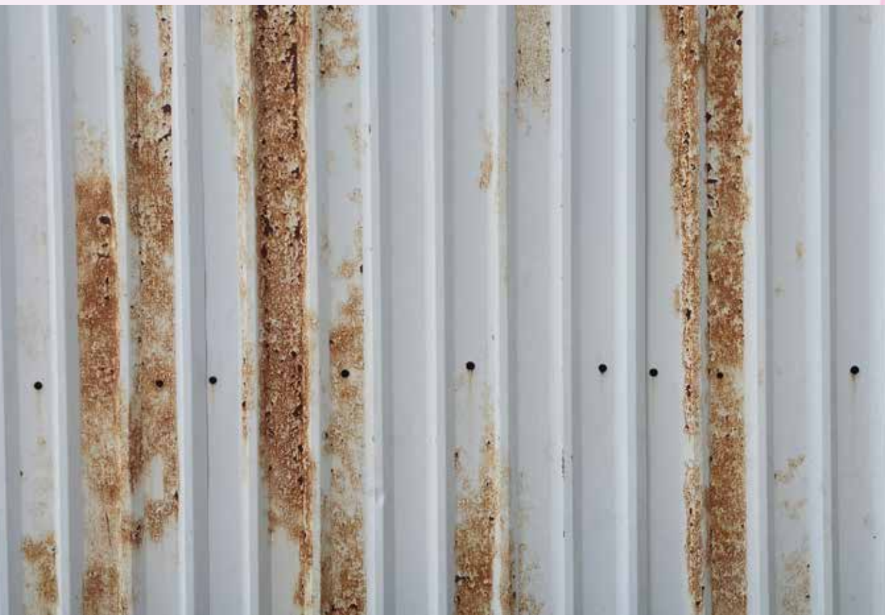
Below: Rusty corrugated sheet metal near a sidewalk.
